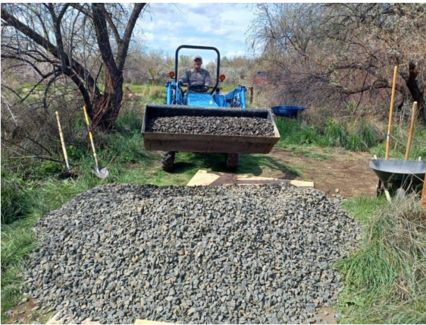
We used our new tractor to position material at the far end of the trail
